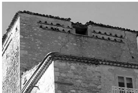
Figure 6 : Earthquake damage to the tower.
